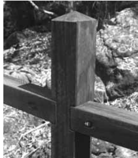
Fig 16 Post projection breaks line of the rail
