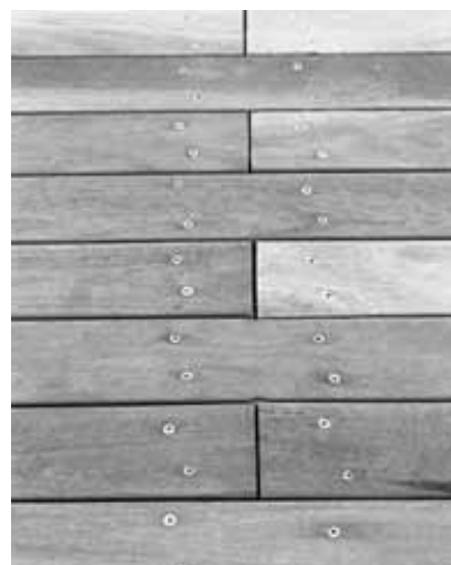
Fig 22 Staggering of plank joins in wide sections of decks is facilitated by paired joists
