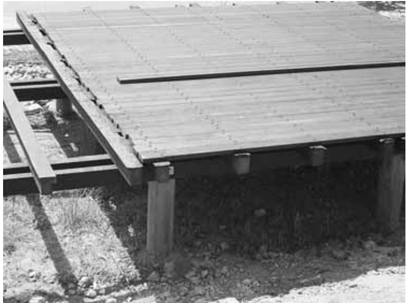
Fig 28 A wide section of deck split into two sections. Note the paired joists. Decking ends are about to be trimmed and a banding plank installed before continuing with the deck.
